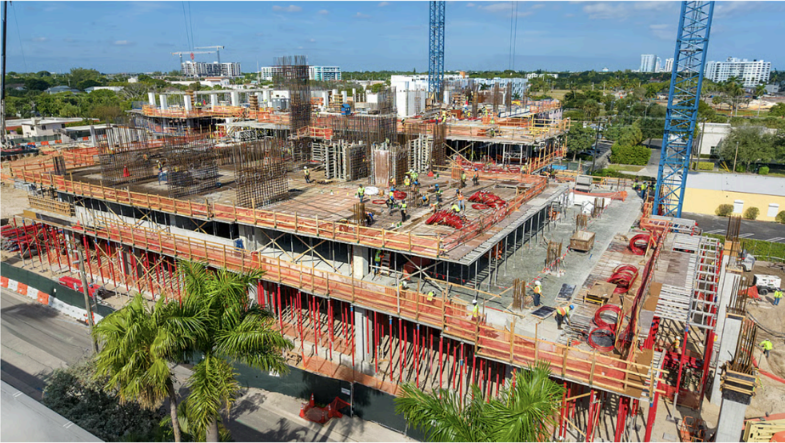
Construction crews advance work at Olara as vertical construction reaches the podium level along the West Palm Beach waterfront Photo Courtesy of Olara
